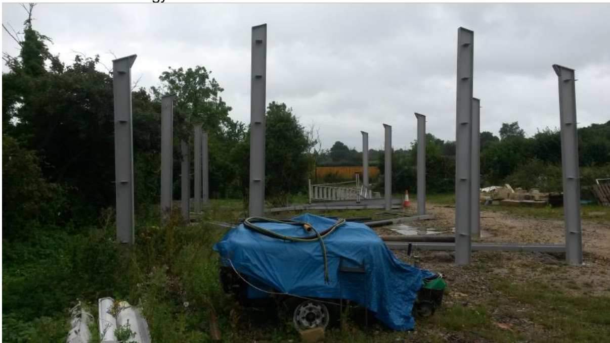
View of the frame of the barn from the southwest adjacent the existing hedgerow boundary
